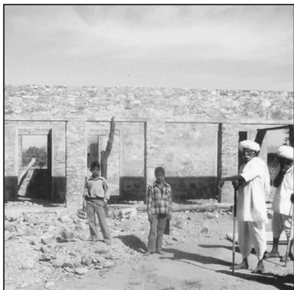
The land donated by Mr. Kalu Ram Yadav on which school building is being constructed
